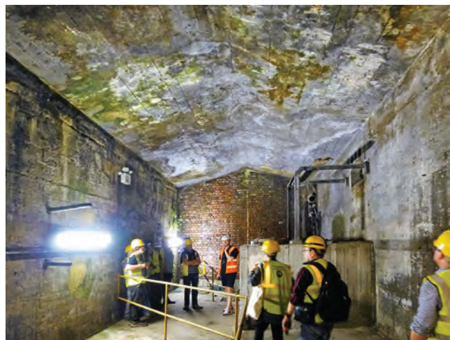
SubBriters looking through the access hatch at the Victorian arches spanning the original George’s Dock.
